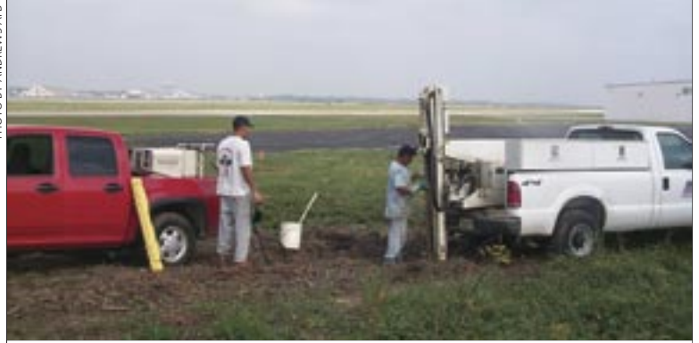
Contractor personnel inject HRC into the ground to enhance the breakdown of carbon tetrachloride.
